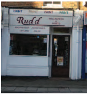
Picture 5.24 9 Whitchurch Lane- Typical original shopfront, with pilasters dividing it from its neighbour
