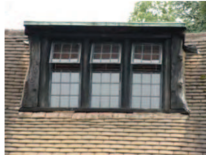
Picture 3.71 Sloping pitched roof dormer to the Tithe Barn, Old Church Lane
