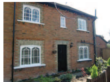
Picture 2.57 No. 12 Green Lane Cottages and its decorative brick quins and brick surrounds to windows
