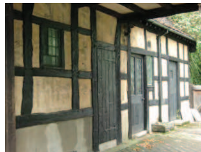
Picture 3.49 Lathe and plaster infill on wall to the grade II listed Cowman's Cottage, Old Church Lane and part of its roof over the carriage-way
