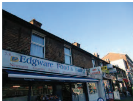
Picture 5.26 Fascia board for nos. 7-8 High Street which cuts across the two units, detracting from the regularity of the terrace
