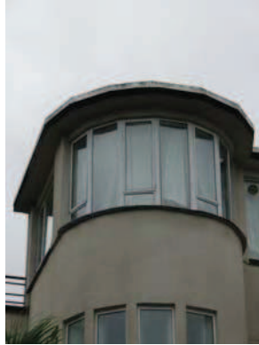
Picture 4.84 Replacement windows here detract from the intended delicate nature of these windows and strong geometrical lines of the building
