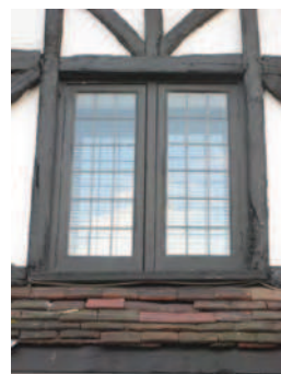
Picture 5.49 Good timber casement leaded light window to nos. 97-101 High Street, Edgware
