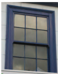
Picture 5.46 Vertical emphasis to first floor windows with this one being a double hung 6 over 6 pane sash window
