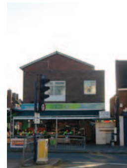
Picture 5.69 Railings around the corner of Edgware Road and Whitchurch Lane are damaged and add clutter to the streetscene
