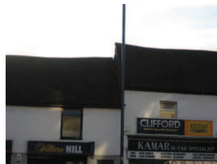
Picture 5.43 Good steeply pitched roofs of no. 83 and no. 85 High Street, Edgware - the slight variation in roof height helps create an interesting roovescape
